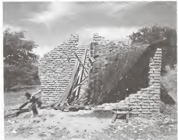
Figure 14. East end of the Kentucky Camp barn. The collapsed roof was acting as a "sail", causing the central partition wall to lean, and was removed by subsequent stabilization efforts. Photo by Jim McDonald.
